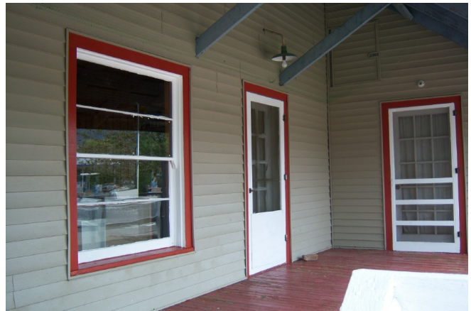
A cleaned up and painted front (Main Street) porch at the Depot.
